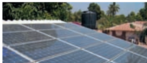
PV generator in Gambia
